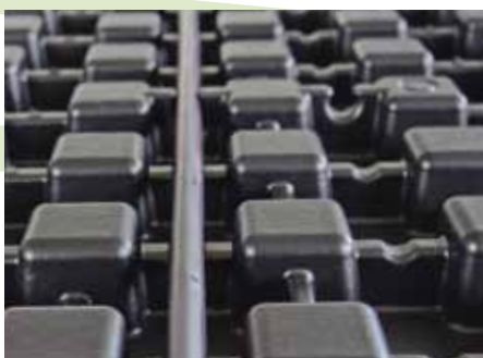
Slotting the dripperlines into place. The lines are then connected to the control system.
